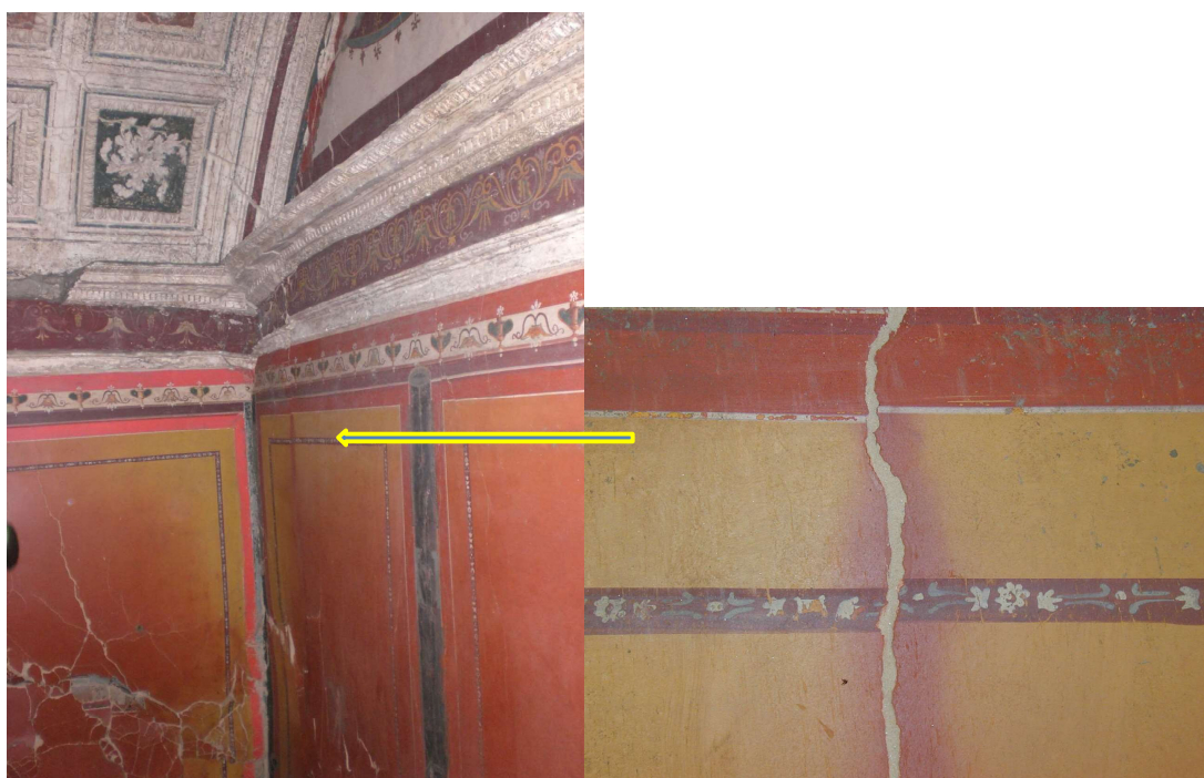
Figure 3. Villa dei Papiri – Ercolano. The effect of the high temperature gas transforming yellow ochre to red ochre is evident. The crack in the wall also points to what happened. (by INO – CRN)
